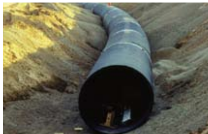
Storm Water Drainage and Retention
